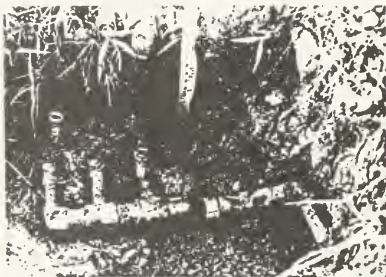
Demolition of Allen Parkway Village has progressed as far as the excavation and disconnection of water pipes in some places.
